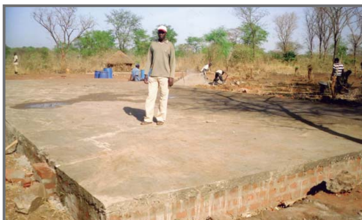
The contractor standing on the foundation of what will be the church building on the campus.
