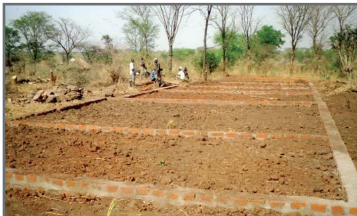
The trenches have been dug, the footing finished and now ready for the concrete foundation. Each of the places where dirt is seen between the footings will be a room of the South Sudan Bible School building.
